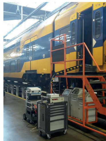
BALTO 6kA system at work at NedTrain
